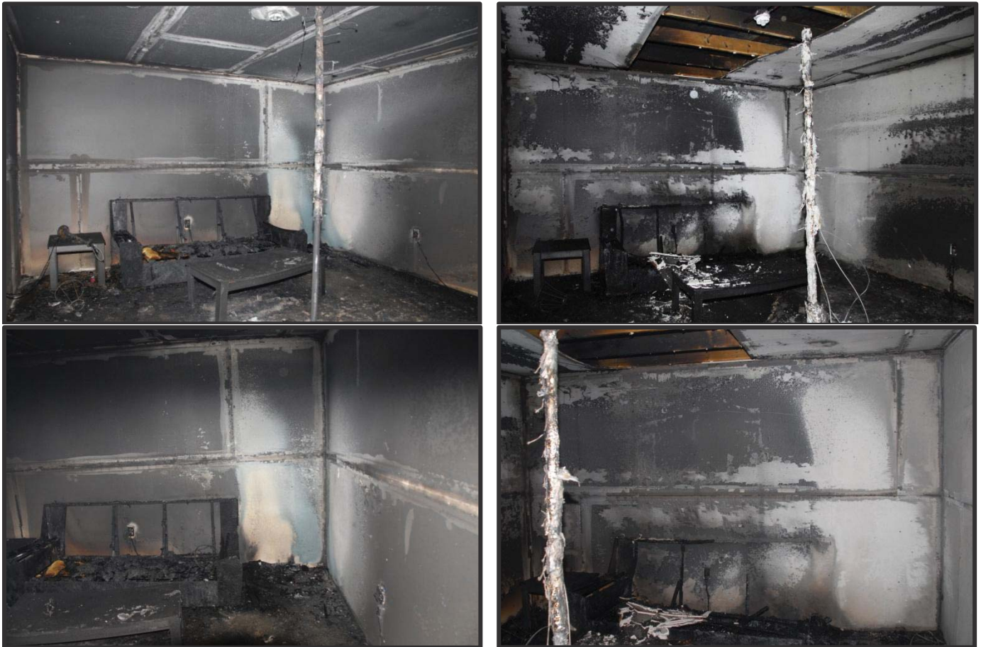
Figure 12: Post-fire Damage-Right End Table=Area of Origin (left) Cell 1; (right) Cell 2
