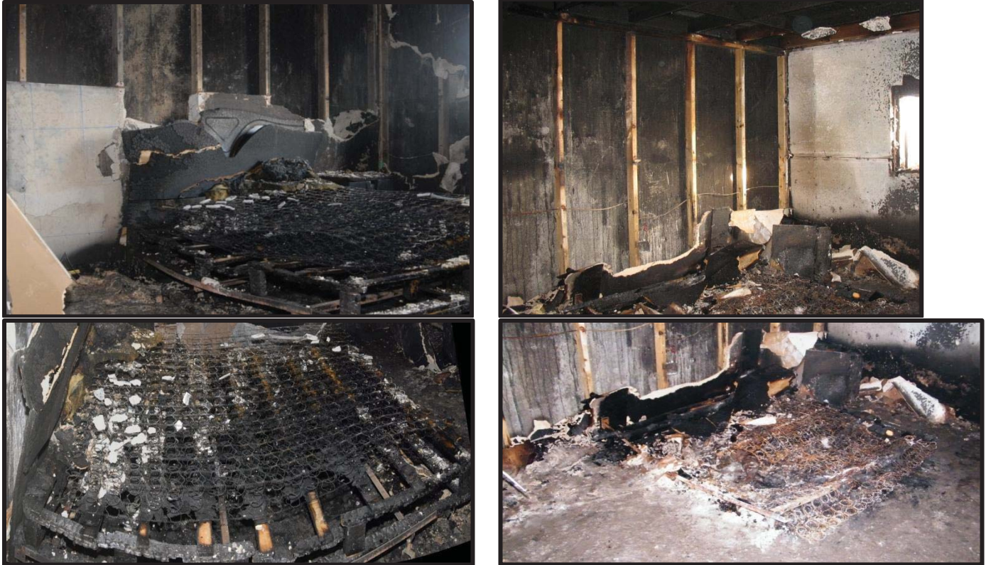
Figure 22: Post-fire Damage (left) Cell 1; (right) Cell 2
