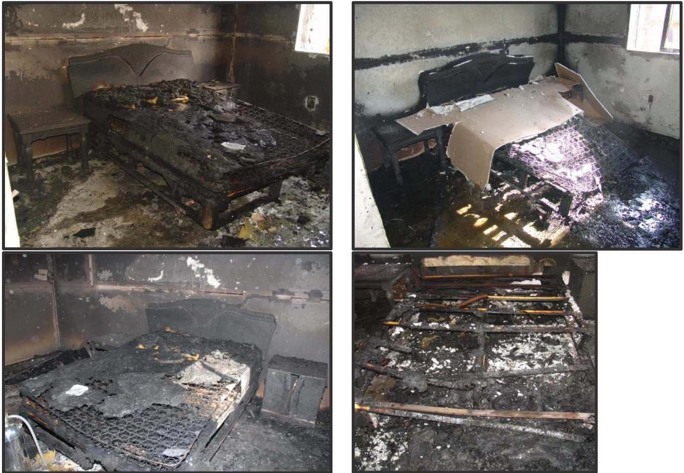
Figure 15: Post-Fire Damage - Foot of bed=Area of Origin (left) Cell 1; (right) Cell 2 (note: drywall from ceiling failed)
