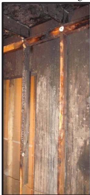
Figure 23: Cell 2 Wood Stud charred behind left nightstand
